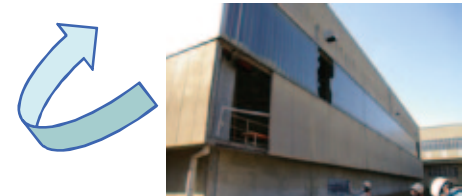
Damages to the multi-purpose gymnasium (at the time of the earthquake)
